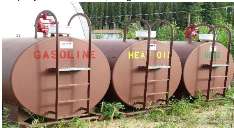
FIGURE 11 FUEL TANKS, PICTURE TAKEN IN HEALY LAKE
